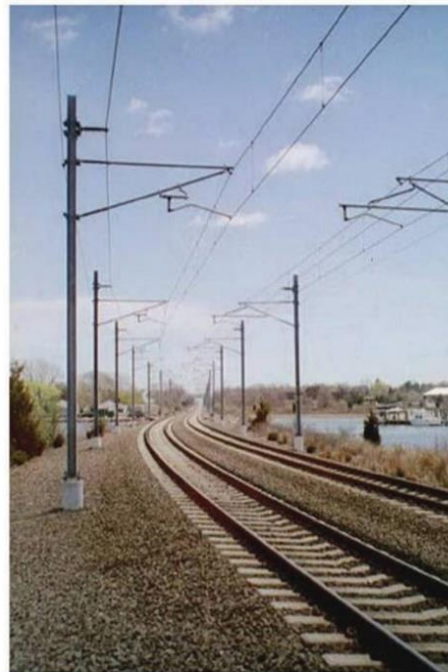
Amtrak's North End Electrification
